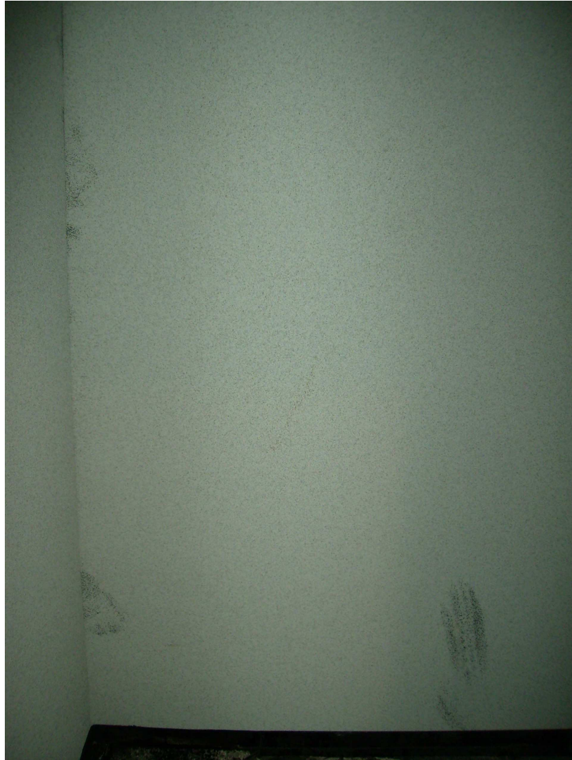
Appearance of the sample before the SBI test (long wing) in accordance with UNE-EN 13823:2002
