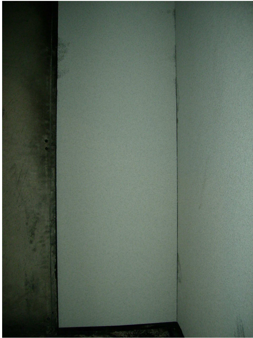
Appearance of the sample before the SBI test (short wing) in accordance with UNE-EN 13823:2002
